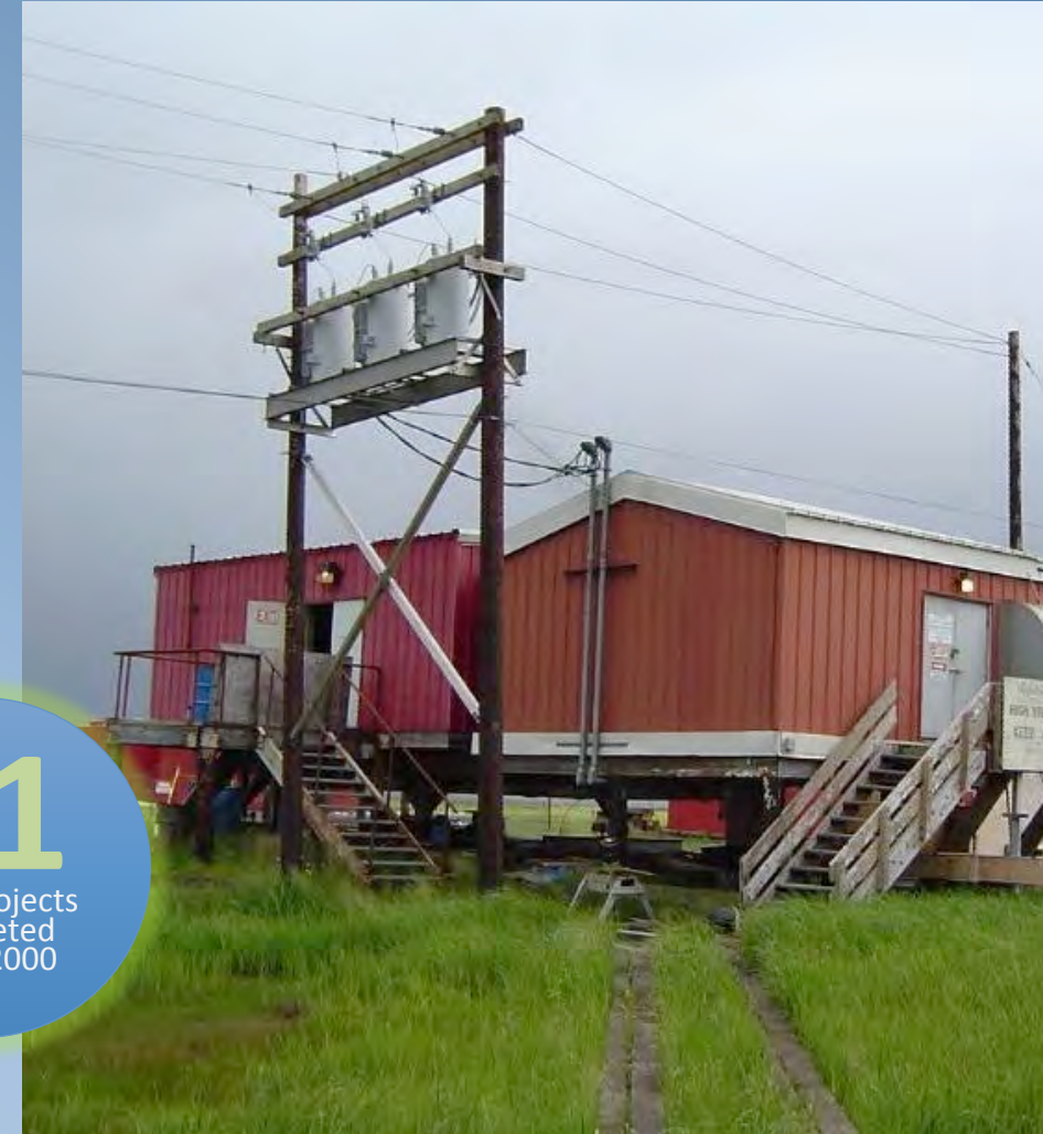
Kipnuk power house in 2004. A new power house module for Kipnuk is currently under construction by AEA contractors.
