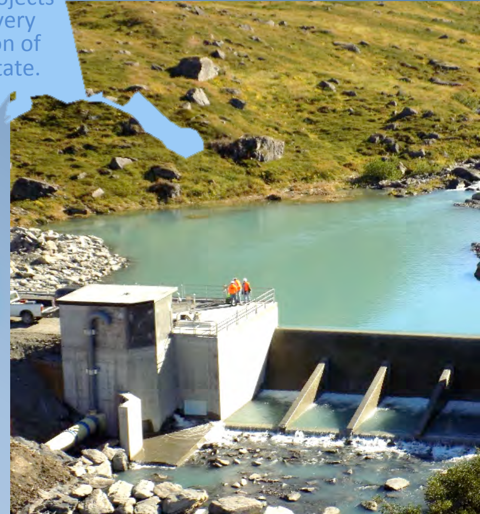
Allison Creek Hydro, Copper Valley Electric Association
