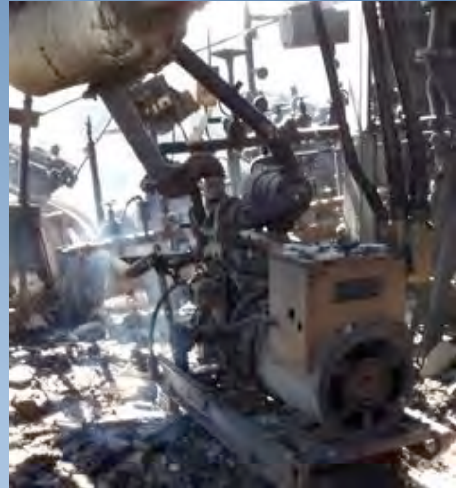
Birch Creek power house fire, 2011
